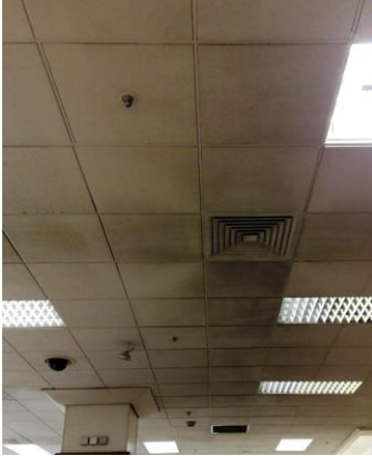
Faded ceiling with soot damage around vents
